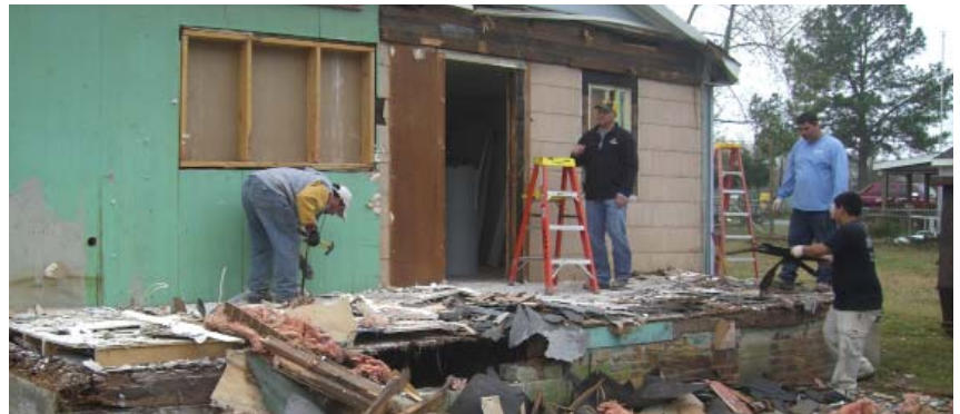
The team gets their hands dirty as they help demolish the backside of a house slated to be Johnston County's Special Olympics main office
